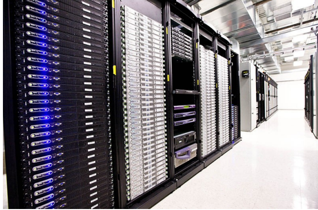
Illustration 1: Illustration 1: This is what the inside of a data center looks like. Somewhere in the world a data center similar to this one is storing a copy of this very document. Photo: Global Access Point, Public Domain
